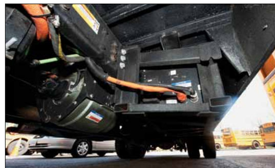
Electric Motor and Battery Pack
