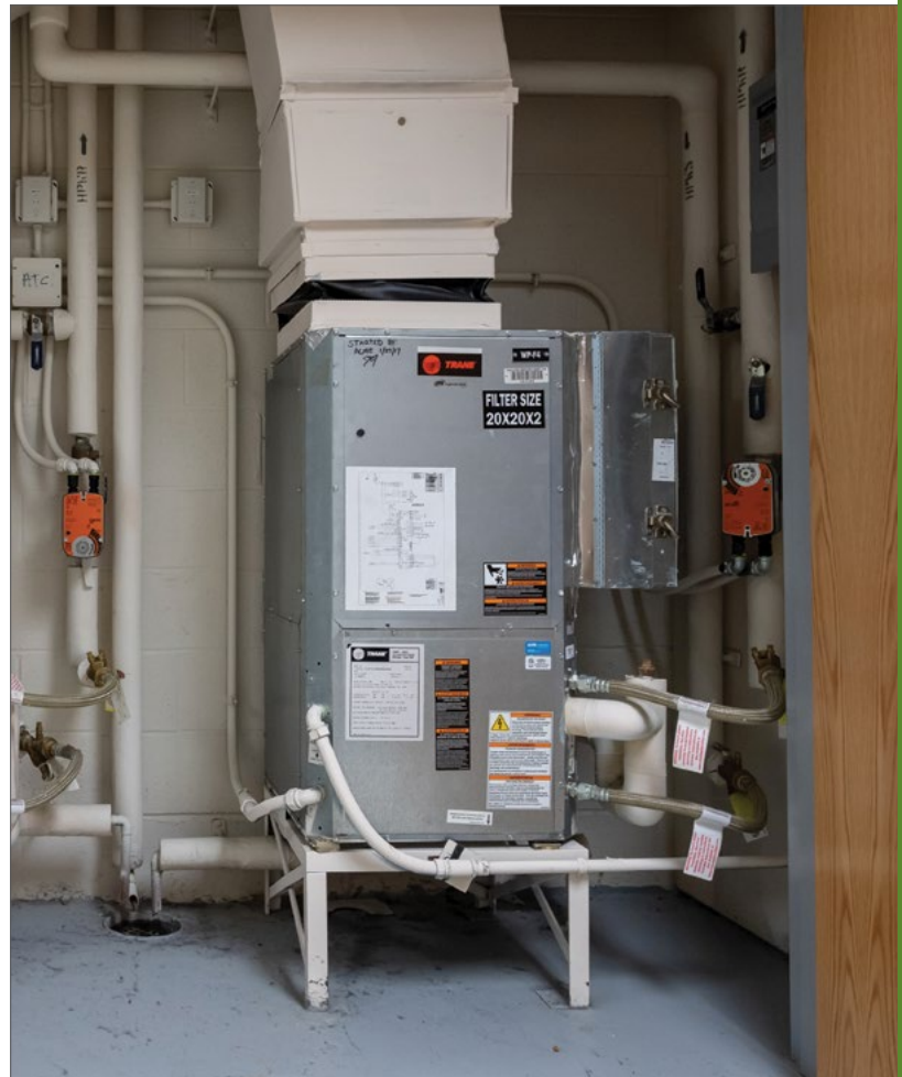
Ground Source Heat Pumps heat and cool using the constant temperature of the earth extracted from wells hundreds of feet deep for the source of heat transfer.
