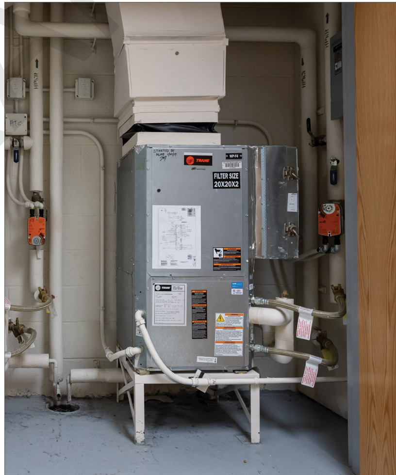
Ground Source Heat Pumps heat and cool using the constant temperature of the earth extracted from wells hundreds of feet deep for the source of heat transfer.
