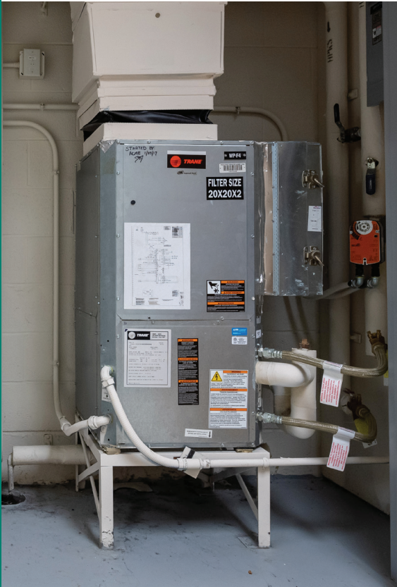
Ground Source Heat Pumps heat and cool using the constant temperature of the earth extracted from wells hundreds of feet deep for the source of heat transfer.
